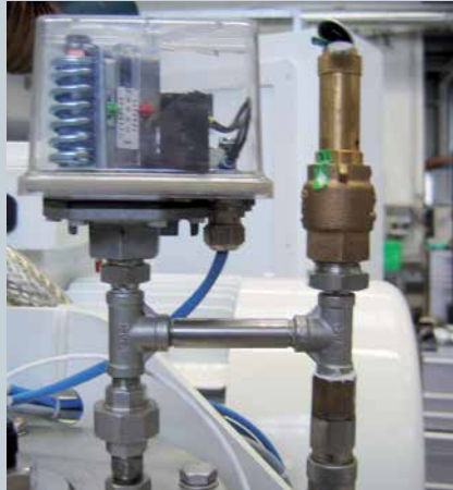
Sealing pressure monitoring
