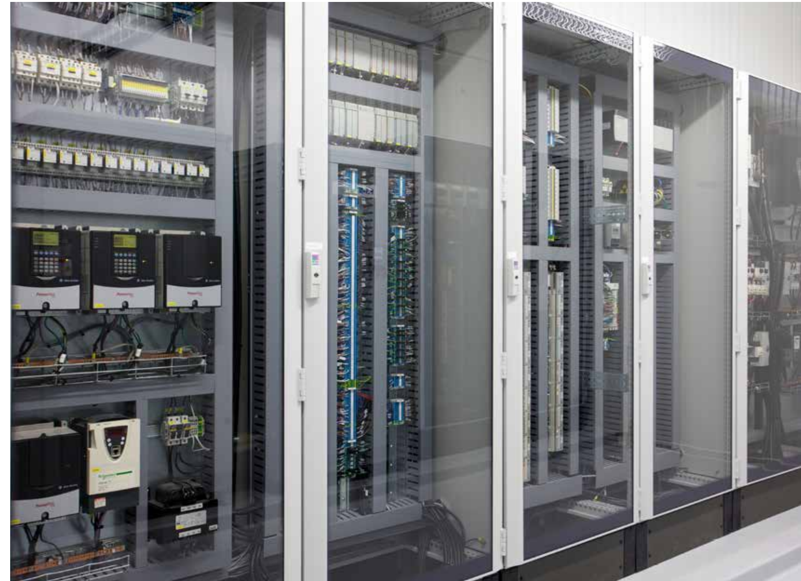
Equipment Control Center.
