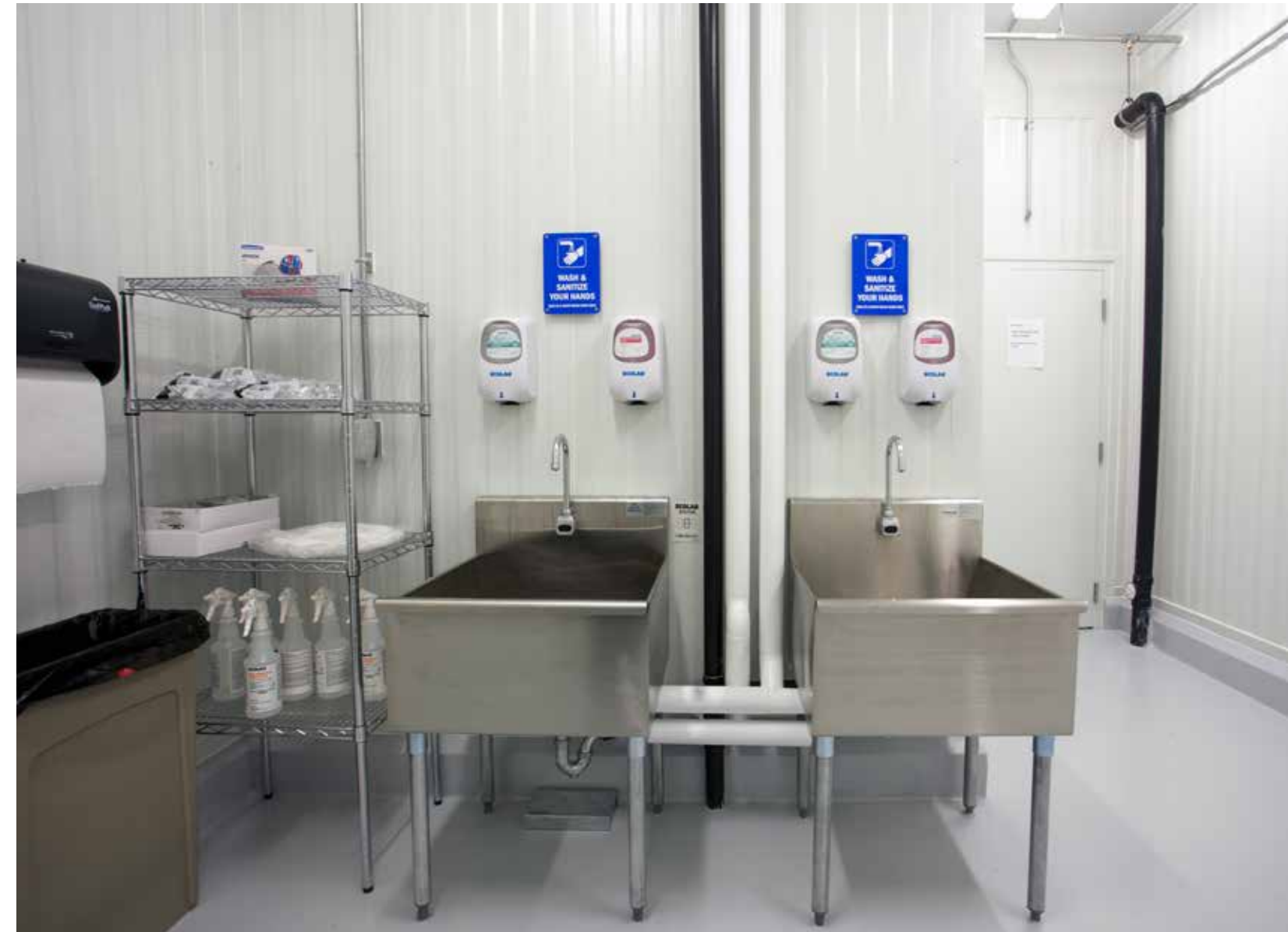
GMP pass-through room.
