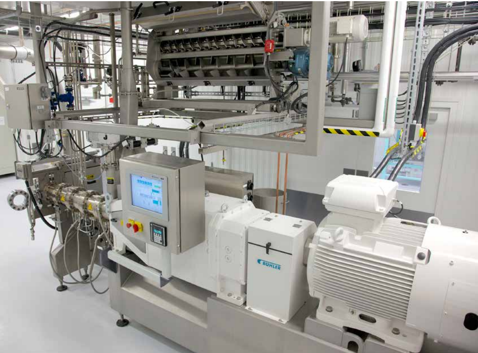
Preconditioning and Extrusion Room.
