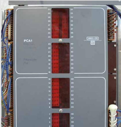
Older Bühler control system SAIA.
