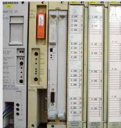
Older Bühler control system S5.
