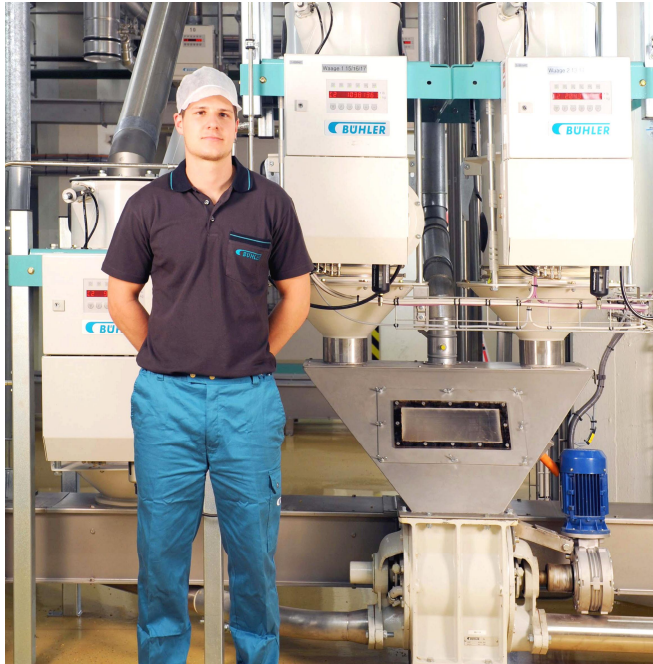
Bühler scale installation
