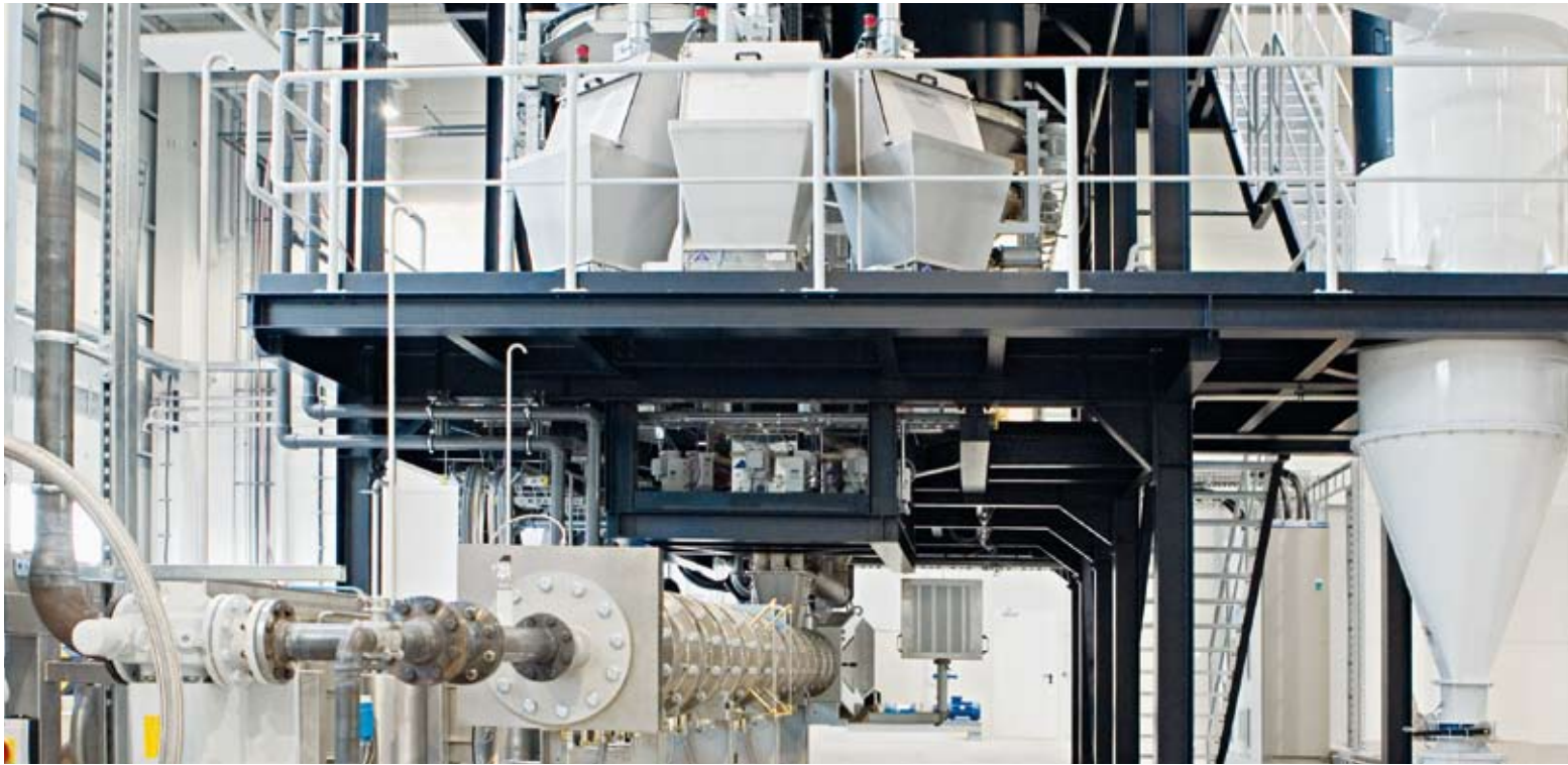
Successful process and project development: Production facility at Schuite & Schuite Druckfarben GmbH – continuous varnish production off 6'000 kilograms per hour, comprised of raw material storage, dosing systems and twin-screw reactor.
